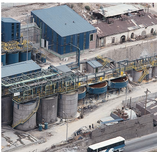
The Tamboraque plant in Peru is currently being recommissioned.
